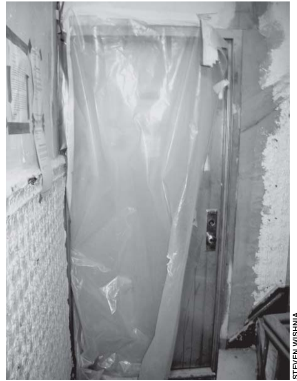
This thin plastic doesn’t keep construction dust out of tenants’ apartments.
