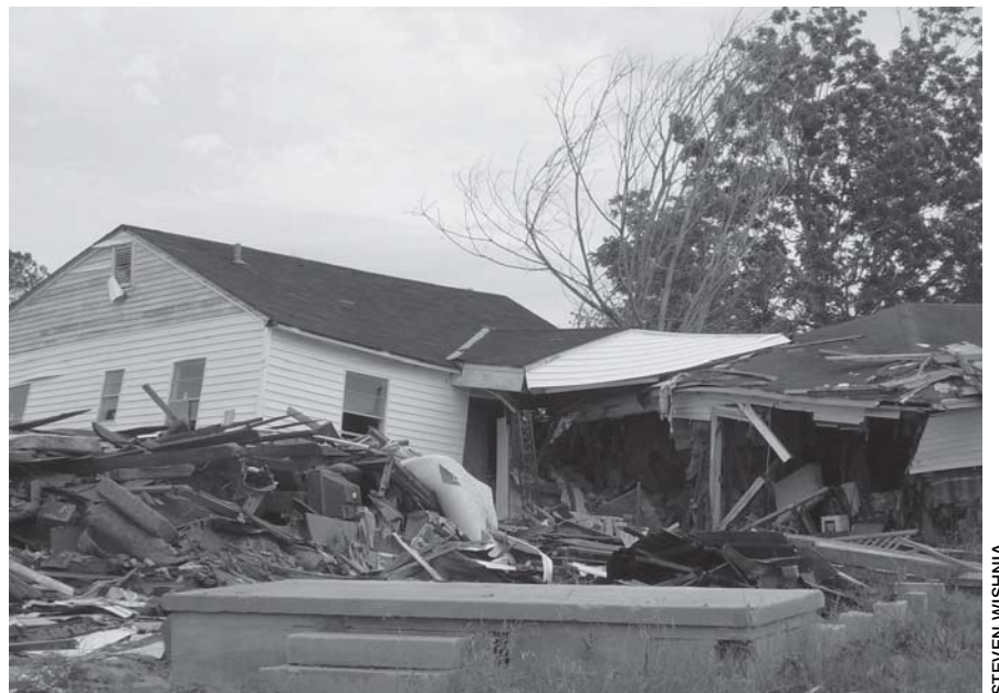
A Lower Ninth Ward house knocked off its foundation by the flood.
